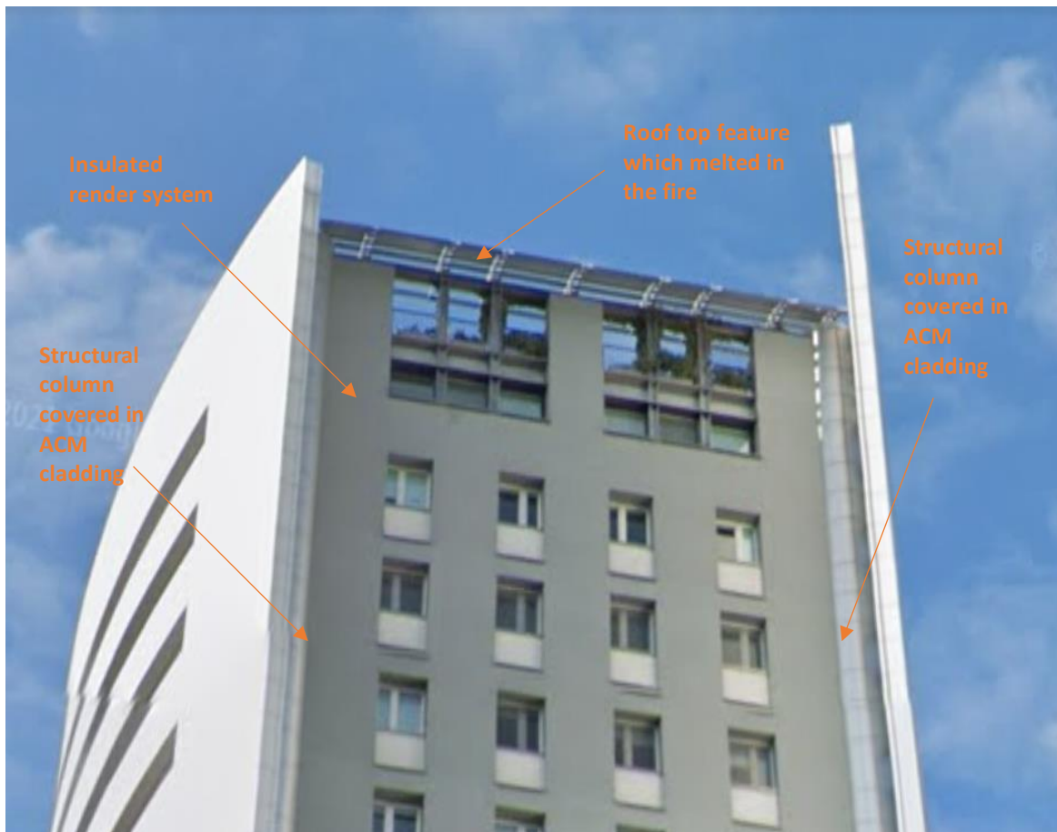
Figure 8: The façade at each end of the building consists of insulated render, but the combustible ACM is in close proximity with the structural columns in direct contact at the interface with the wall. It can also be seen in this photo that there is a feature at roof level which appears to be made of metal, although confirmation would be necessary. This sustained damage during the fire.
