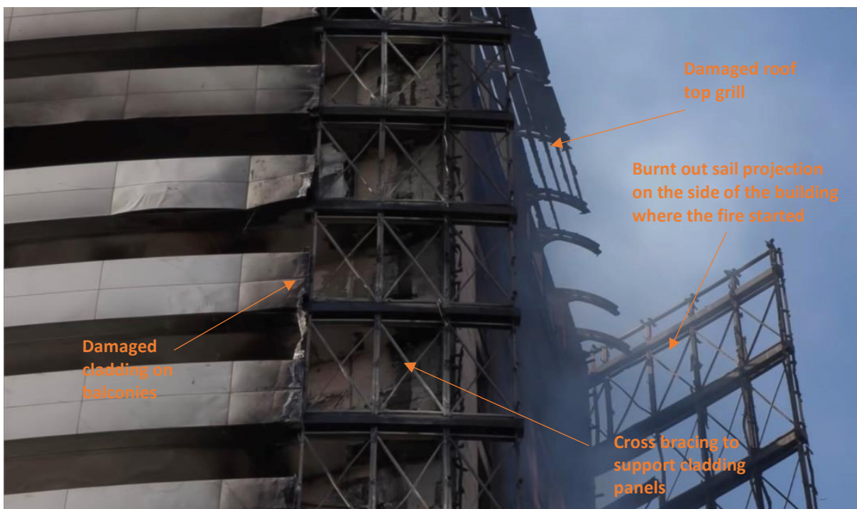
Figure 14: A close up view of the building from the opposite side to that where the fire started; the end of the sail has borne the brunt of the fire with only the framework surviving. It can be seen that the fire stopped abruptly before the balconies, where the cladding has started to delaminate and deform. This suggests that there may have been fire barriers between the balconies and the ends of the sails.
