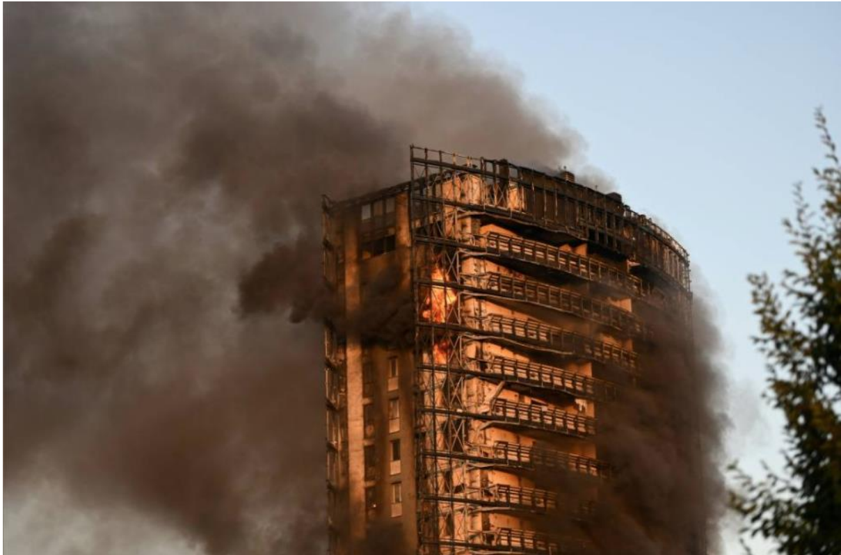
Figure 13: The fire has consumed all of the sail on the south-western side, leaving behind a skeletal framework. It seems that the fire spread along combustible material at roof level to reach the sail on the opposite side of the building.
