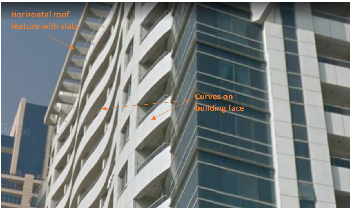
Figure 8: This view is taken midway up the building and is taken from a corner so that an end elevation and a side elevation can be seen simultaneously. The vertical bands of cladding which form balcony walls with multiple ledges would be a means of fire spread, as would the projecting roof-top feature. Photo: The Author
