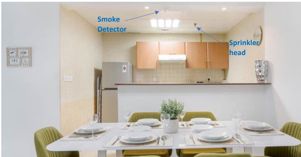
Figure 24: The kitchen and dining area in a two-bedroomed flat of the same plan (but in reverse) as the one where the fire started. There is a smoke detector and a sprinkler head. These provisions are only found in the kitchen and not elsewhere in the flat. Photo: Kennedy Towers www.kennedytowers.com
