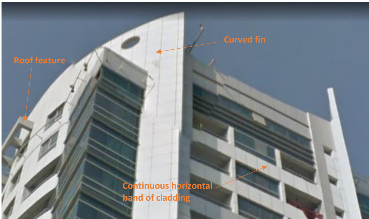
Figure 6: A view of the top of the building showing the curvature of the building face with the projecting fins which curve around the ends of the building at this level. These present a significant fire hazard.
