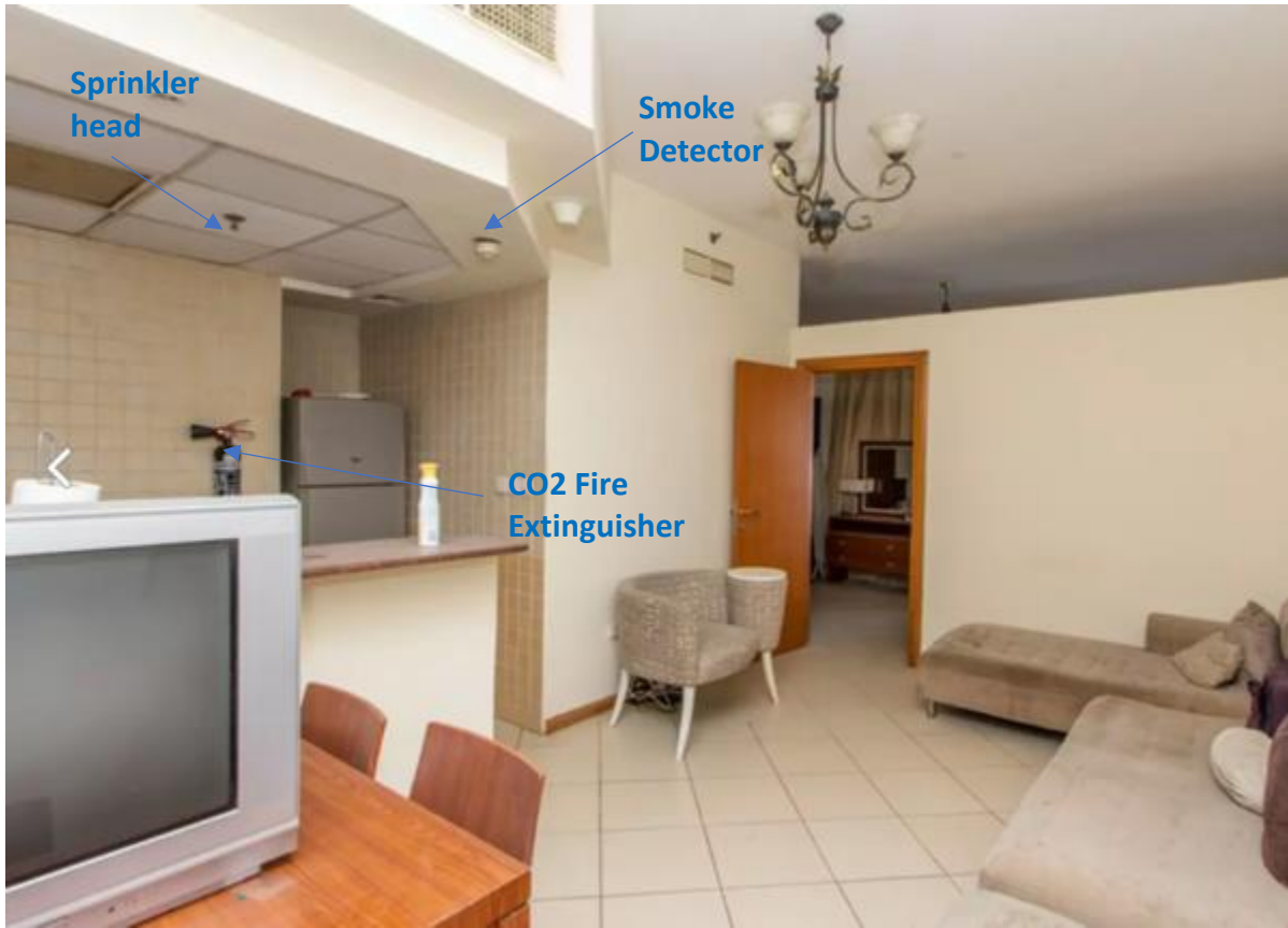
Figure 23: The interior of a one-bedroomed flat in the Marina Diamond 2 building, which has an open plan kitchen/diner/living area. A fire extinguisher, sprinkler head and smoke detector are visible. Such provisions do not appear to be anywhere else within the flat other than the kitchen. Photo: www.bayut.com
