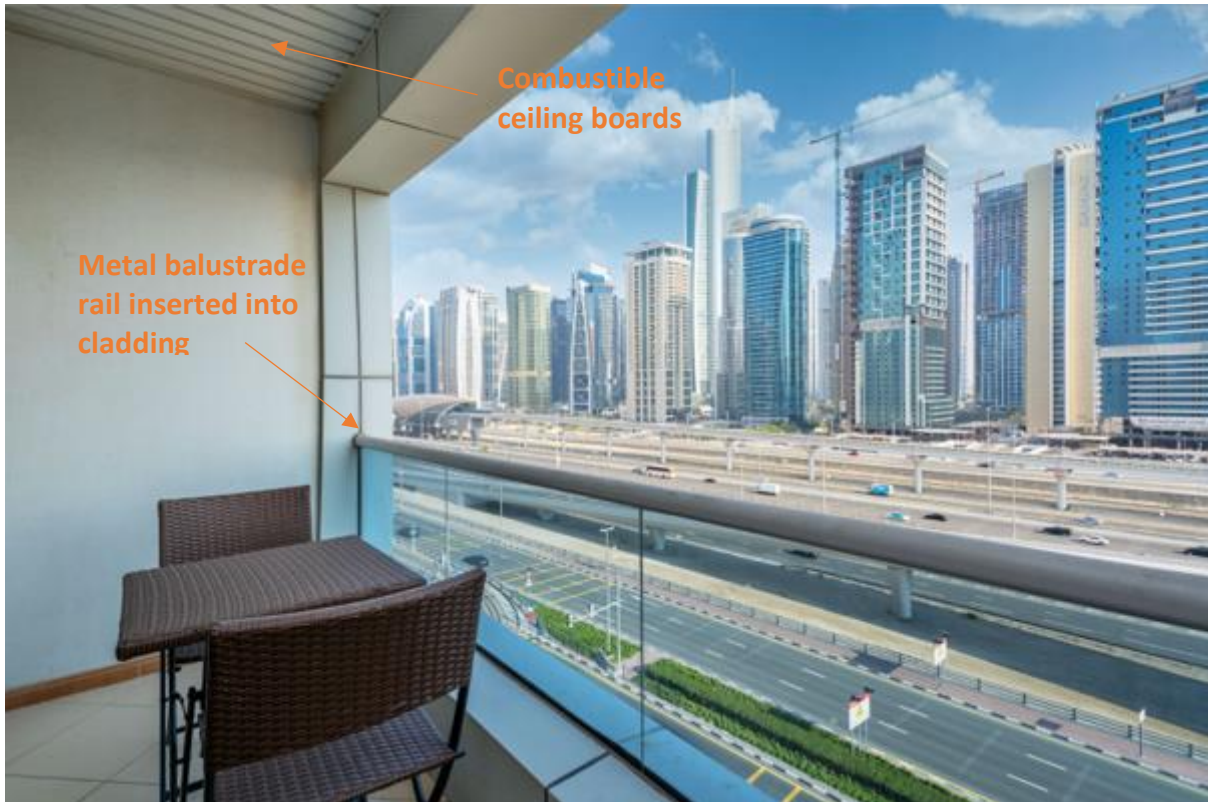
Figure 14: The impressive view from a balcony of a two-bedroomed apartment at the south-east end of the building. This elevation is identical to the one where the fire occurred at the north-west end of the building.
