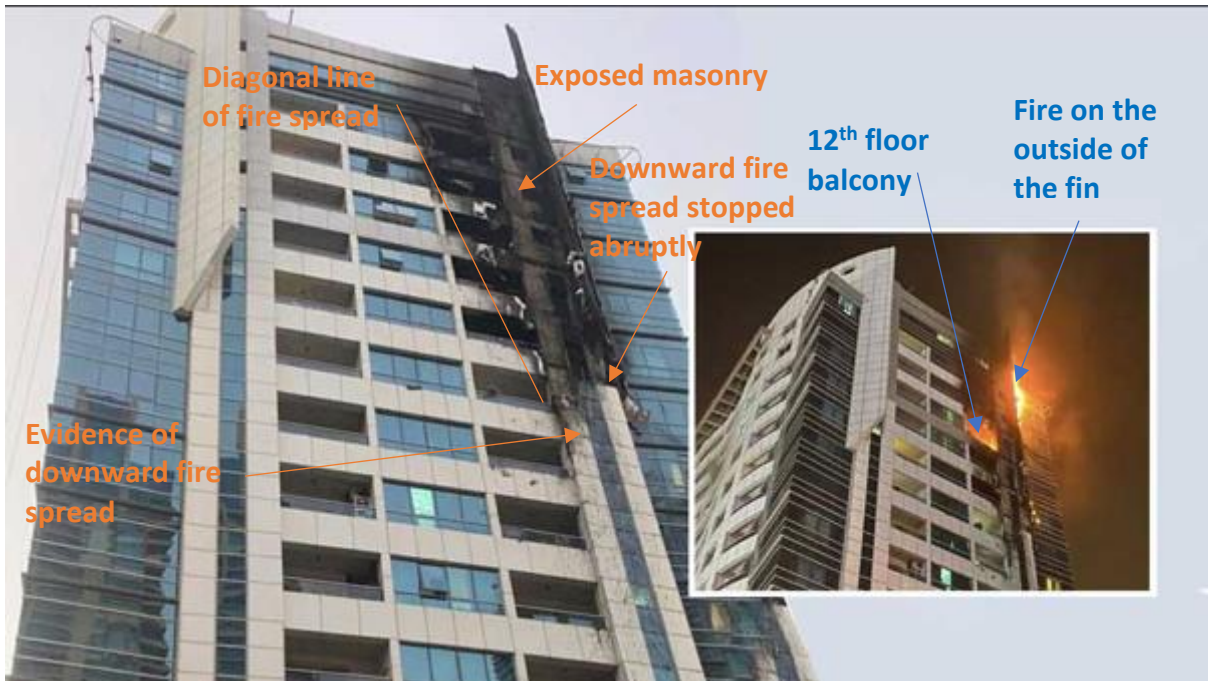
Figure 11 (above, p.15 and below): Two comparable photos showing the building during the fire and the damage which was visible once the fire had been extinguished. Such was the intensity of the fire, especially behind the fin, that the cladding has been completely consumed to expose the masonry behind. Some of the cladding also detached and fell from the building as it burned. Photos: Dubai Civil Defence
