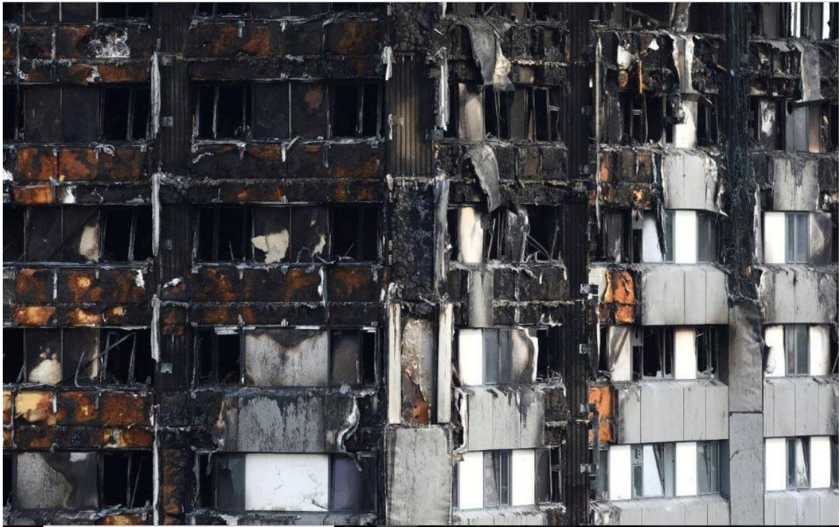
Photo 10: A close-up of the north-west corner of Grenfell Tower showing damaged PIR insulation where the charred layer has detached to expose the material underneath. At these lower levels, the heat was less intense so the insulation has not completely burned through as it has on the upper levels.
