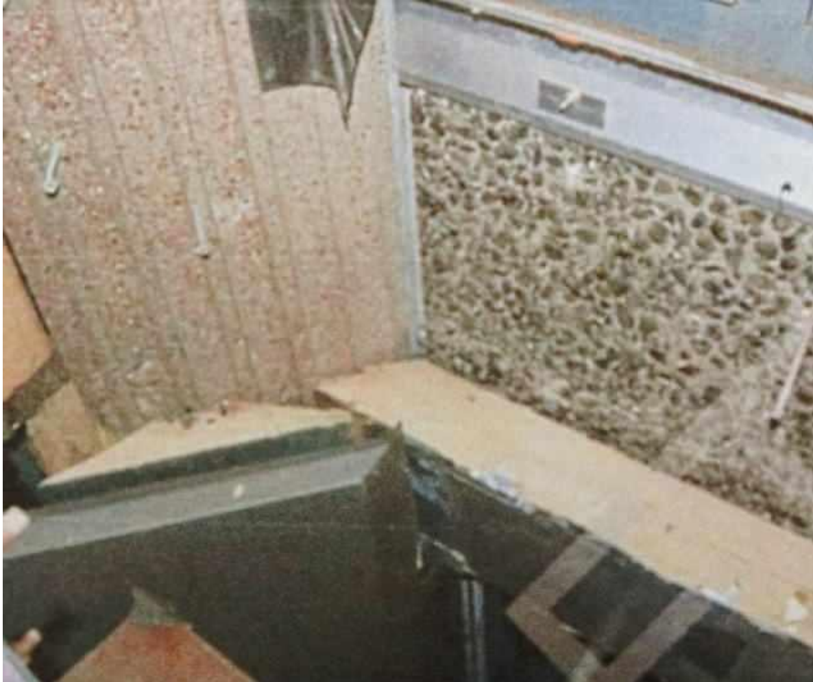
Photo 4: This photo shows the cladding system on one of the lower floors of the Tower. As in Photo 3, the insulation has been poorly cut and the piece on the column does not sit flush against that on the spandrel
