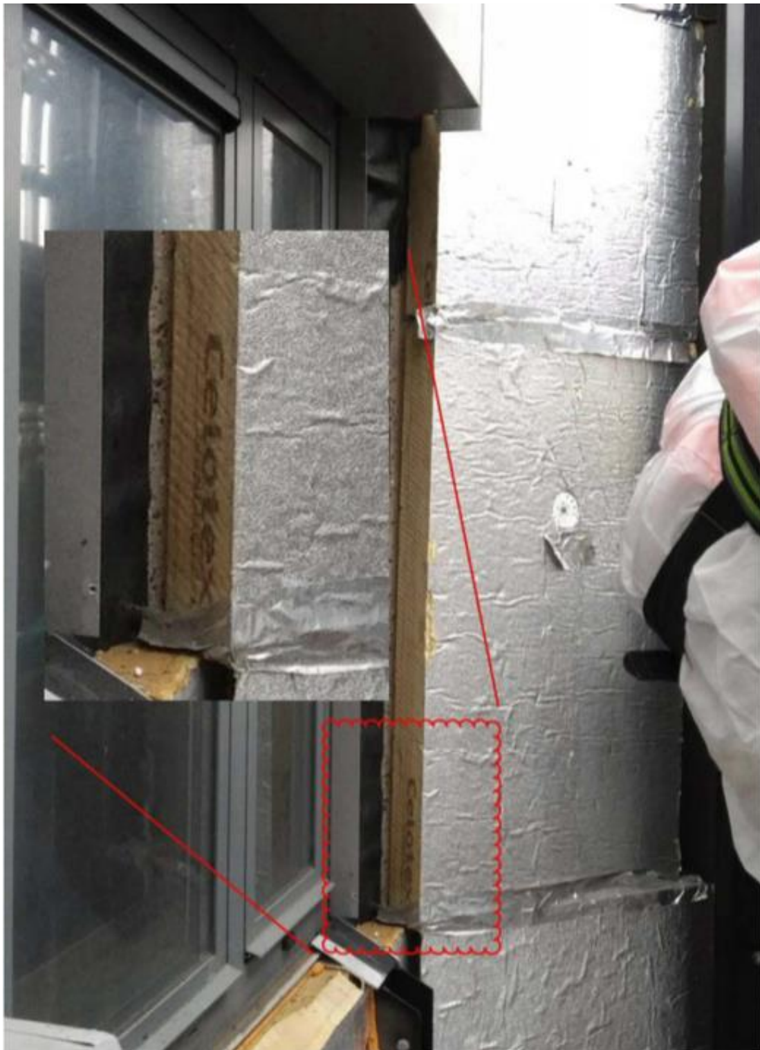
Photo 7: In this photo it can clearly be seen how awkwardly the cladding fits around the columns, and by its sheer bulk, it is difficult to keep it clear of the window opening. It can be appreciated how difficult it would have been to size up the width of the windows accurately and avoid the dangerous gap which was created at the jamb. Photo: Dr Barbara Lane's Supplementary Report, Part 8
