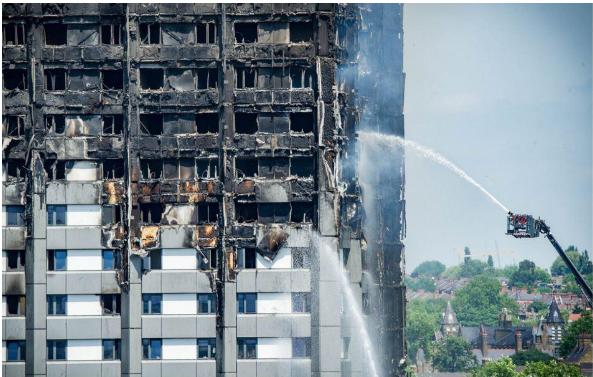
Photo 11: The south face of Grenfell Tower showing the progressive change in the severity of damage to the PIR insulation with ascension up the façade
