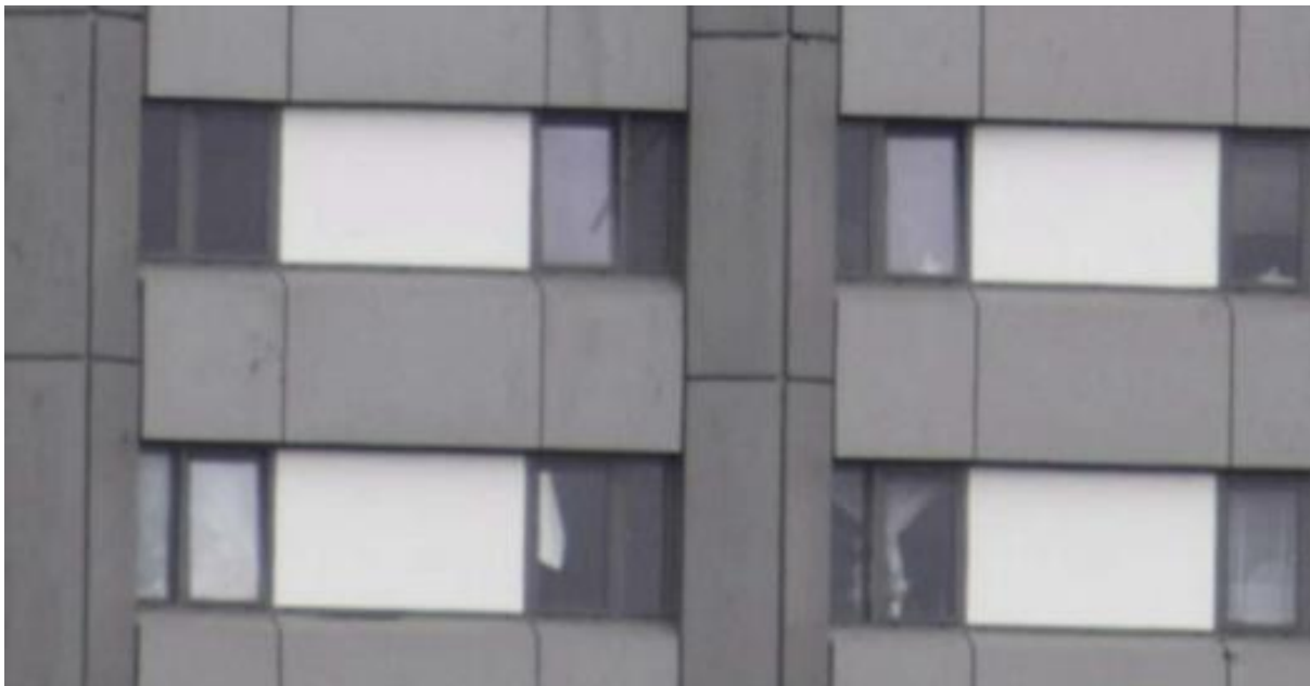
Photo 5: A close-up view of Grenfell Tower showing windows which have been opened using the “tilt” option. They are tilted inwards along their bottom edge.
