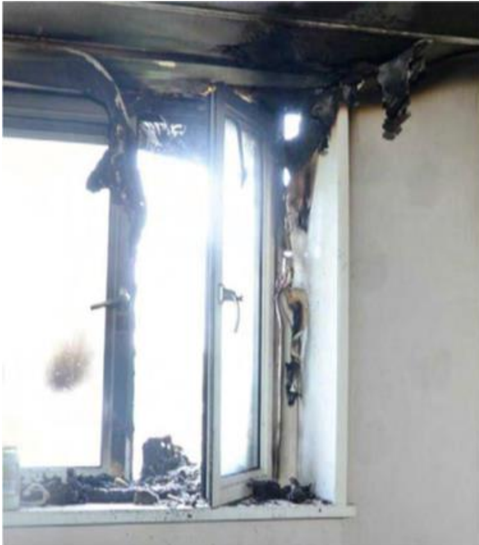
Photo 6: A fire damaged window viewed from the inside which has been opened using the “turn” option to disengage the tilt mechanism and allow it to be fully opened as a side-hinged casement.
